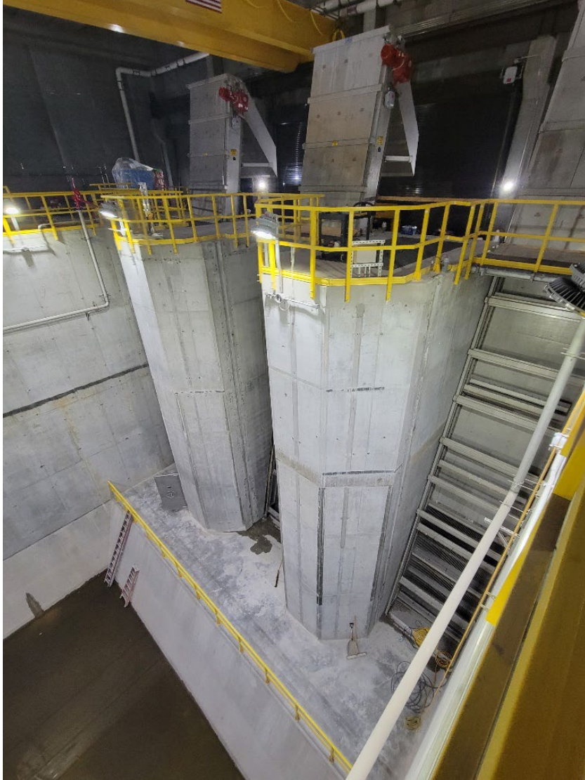
Picture 1 Headworks/Screening Area
